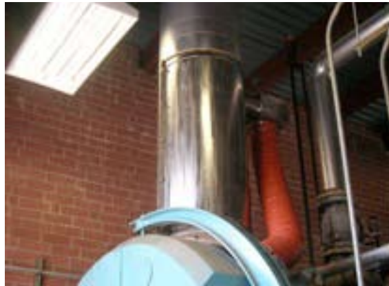
The Mega combustion air pre-heater installed on a 300HP boiler
