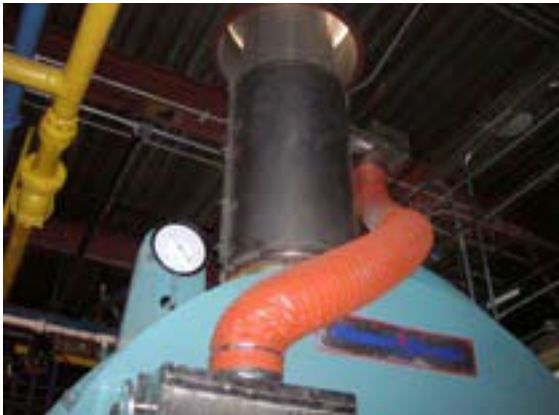
The Mega combustion air pre-heater installed on a 600HP boiler
